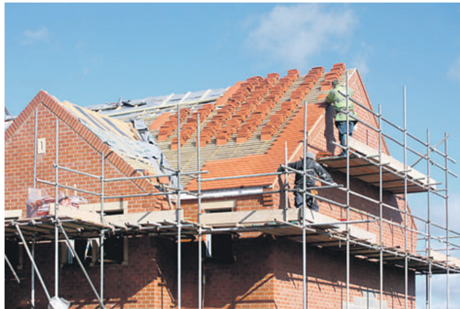
NEW HOMES: Found to have problems with infrastructure and construction.
