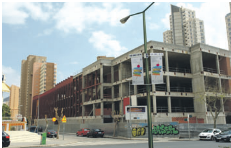
BUILDING WORK: On the unfinished Benidorm Cultural Centre is about to restart.
