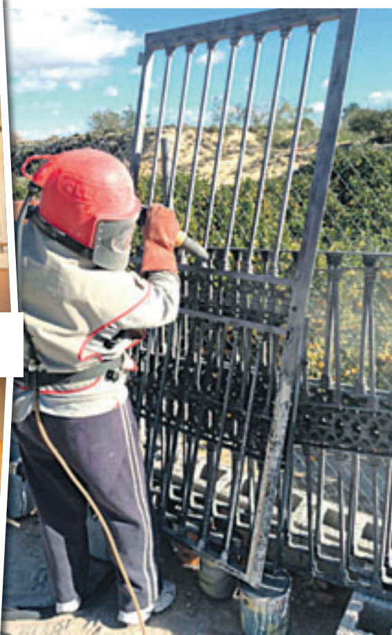
SAFETY FIRST: Make your grill a security grill to allow for exit in an emergency.
