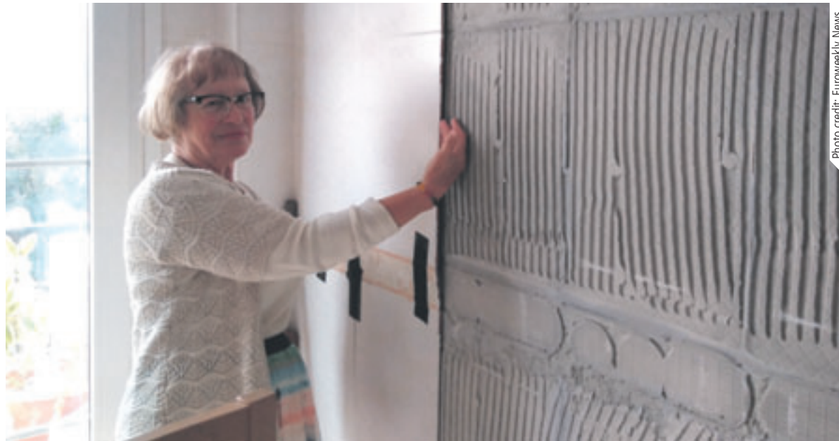
JANET HAYDEN: Shows the damage to her home.
