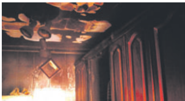
DAMAGED FLAT: Fortunately there were no injuries.
