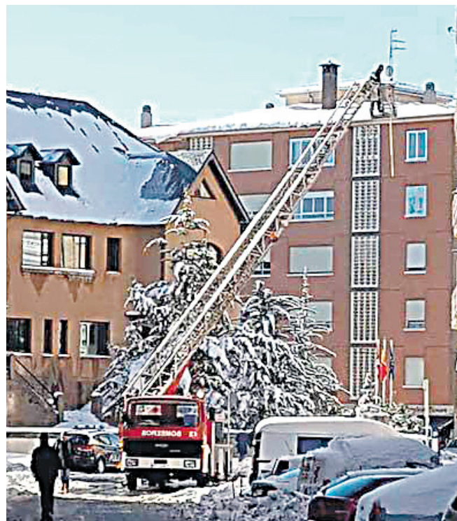
ICICLES: Fireman have been working to clear roof tops.
