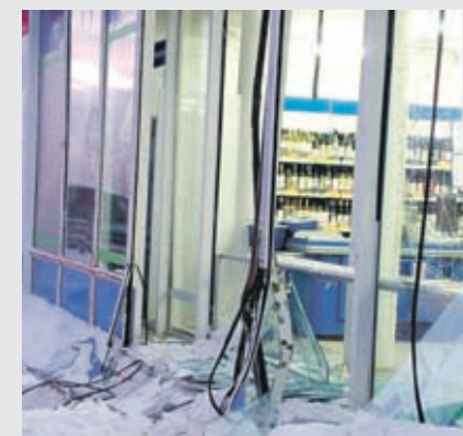
WRECKED: The supermarket window demolished by the tank.
