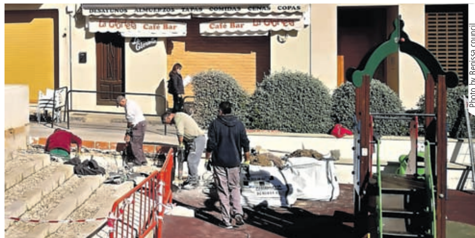
PUBLIC FACILITY: The building of the new toilet has begun in Benissa.
