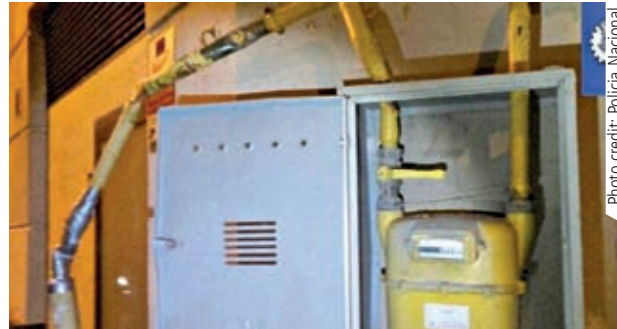
WATER METER: Was stolen from Calle San Jose.
