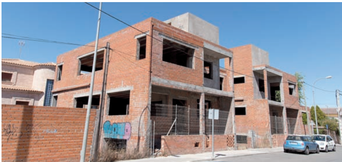
BUILDING BLOCK: The housing crash left Sesena littered with unfinished homes.
