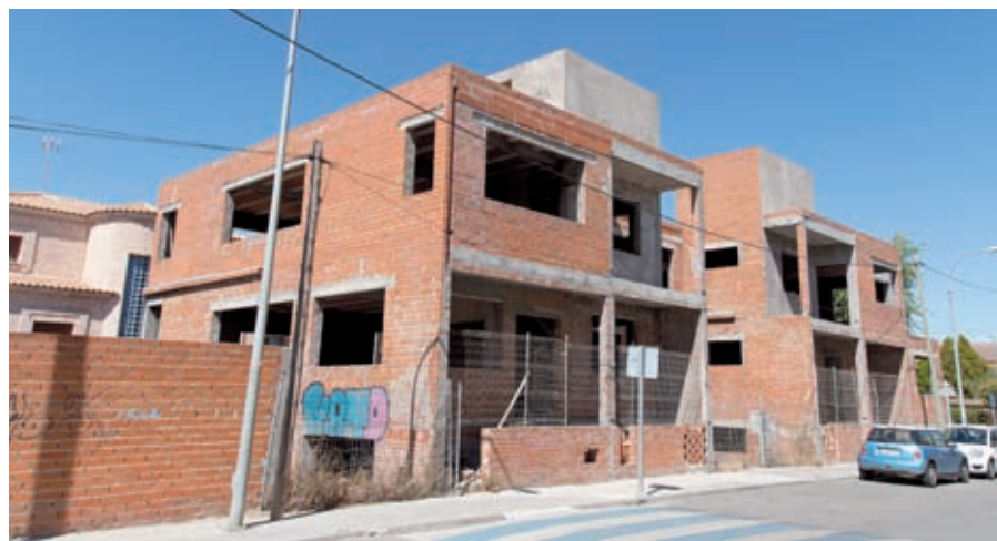
BUILDING BLOCK: The housing crash left Sesena littered with unfinished homes.
