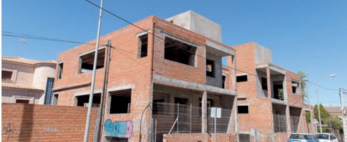
BUILDING BLOCK: The housing crash left Sesena littered with unfinished homes.
