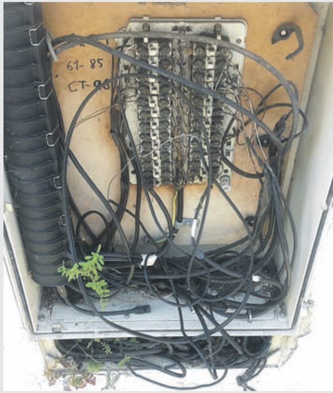
JUNCTION BOX: Open to the elements for three years.
